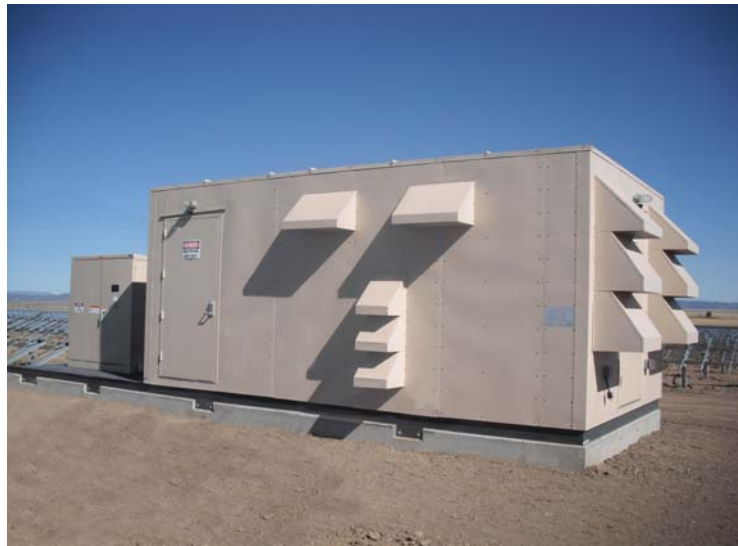
Figure 2-2 Representative Power Conversion Station Photograph
