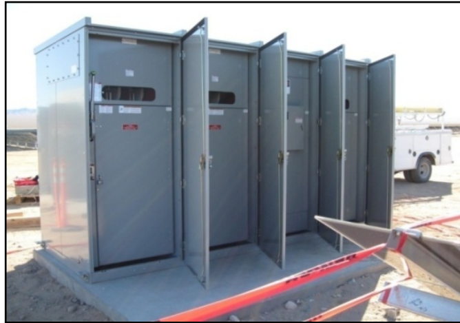
Figure 2-3 Representative PV Combining Switchgear Photograph
